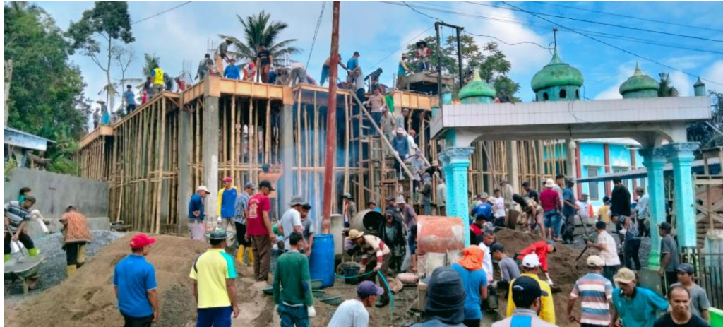
Figure 2 People working together to help rebuild the Muslimin Mosque in Jorong Kayu Tanam, Nagari Labuah Gunuang. Source:Haluan, 2023.
